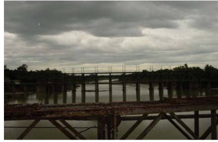
Figure 3. Station 2 (Bulabog-Putian Moroboro Station). View of the dam and impounded water from the upstream hanging bridge in Dingle, Iloilo.
